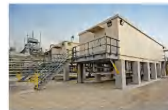
Remote Instrument Enclosures Increasingly Being Used in Process Plants to Save Time and Engineering Costs (Source: Siemens)
